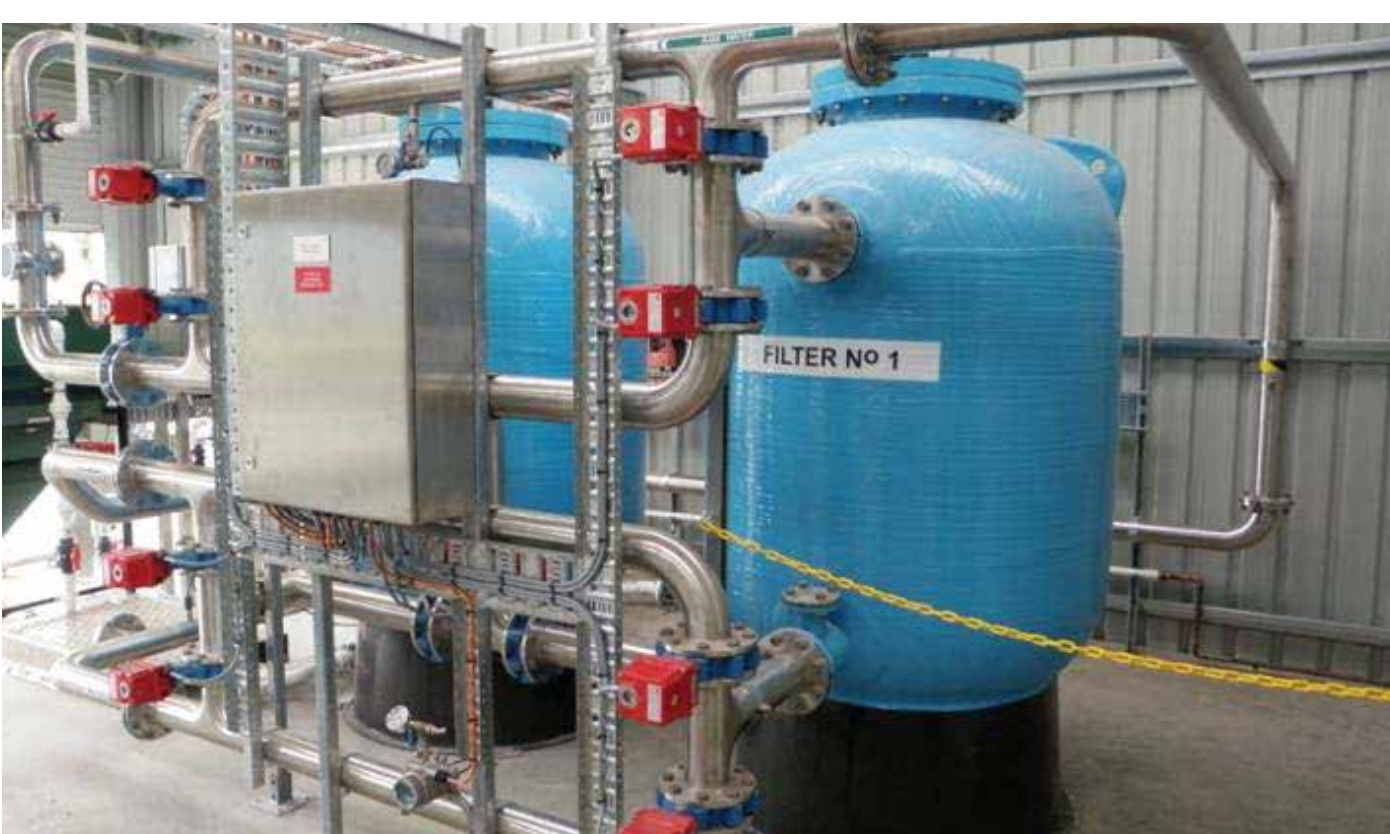
Figure 1: WTP filter cells with manifolds
