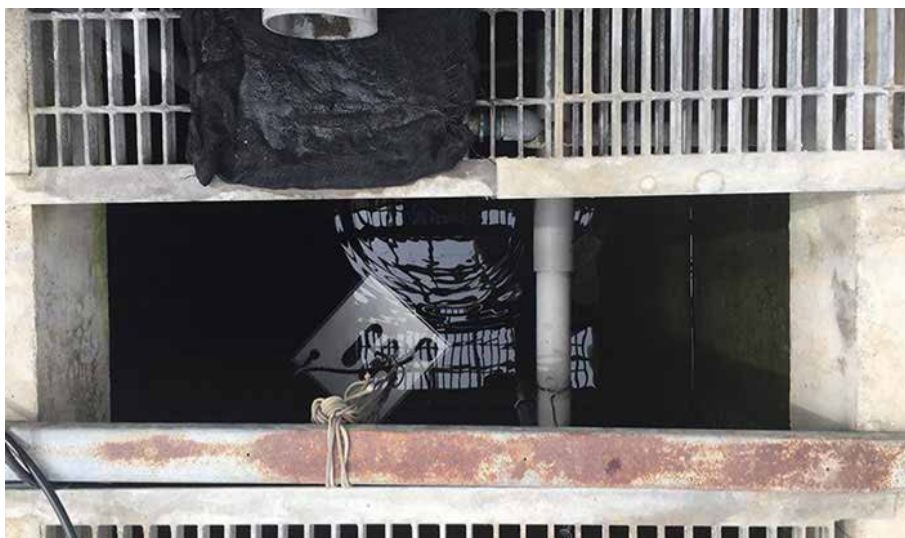
Solari Submersible Ultrafine Bubble generator in irrigation tank at greenhouse site.
