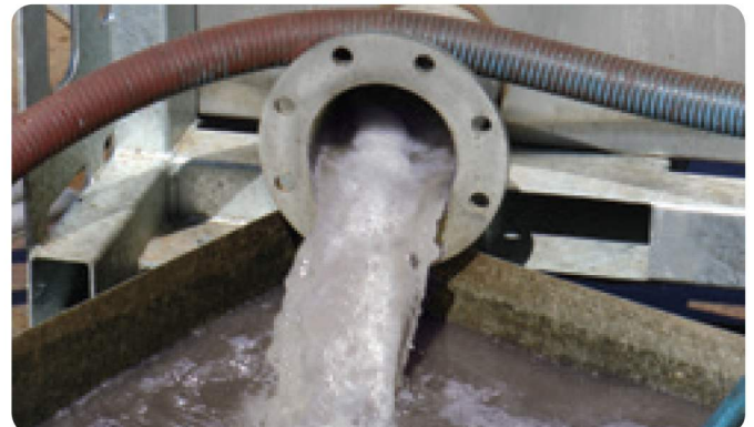
Fig 4. Filtrate being discharged from the Z300A unit.
